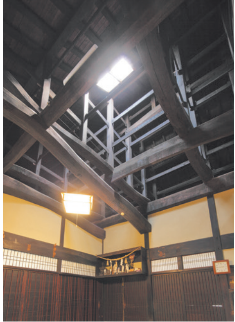
Attic with penetrating tie beams and vertical struts, and glass tile skylight
