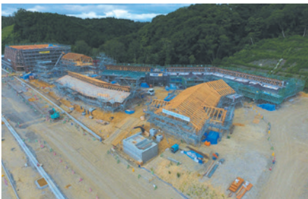
Construction of the school on a wide, elevated site: classroom building (back right), special-purpose classroom building (back middle), indoor sports hall (back left), administration building (right front), and library (middle front)
